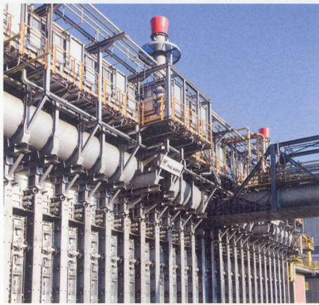
Cover photo: Battery No. 3 at Zentralkokerei Saar, Dillingen, Germany
