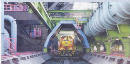
Railway bunker unit with dust capturing hood
