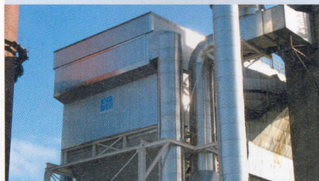
High-efficient bag filter plant
