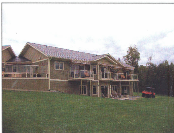
They look like slate but the shingles on this house are made of recycled rubber and plastic.
