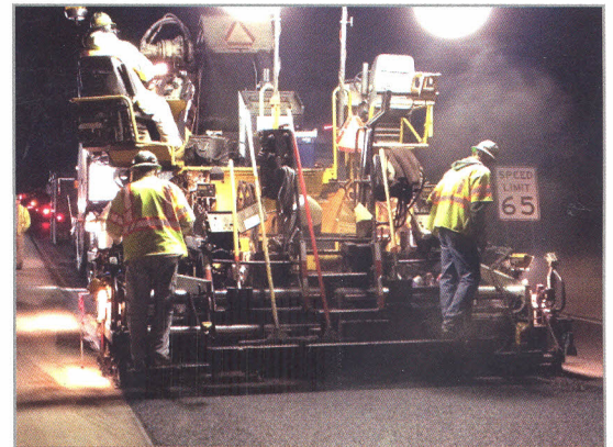
Rubberized asphalt being placed on the wearing course of I-78 in Pennsylvania.
