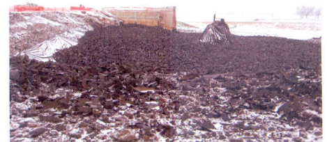
The equivalent of about 820,000 vehicle tires was used to correct poor soils in the Blue Earth County CSAH12 bridge embankment project.
