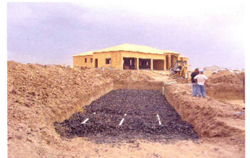
Alabama is the latest in a list of states advancing the use of TDA as drainage media in septic systems. The photo above shows TDA being installed at a Colorado residence.
