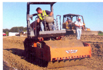
Highway workers are using a mixture of tire shreds and sand in road construction projects that have saved the state more than $1 million over the last two years.
