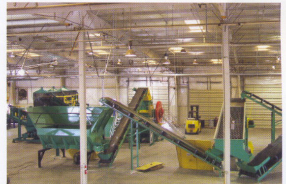
Columbus McKinnon Corp. installed the first complete front-end system for a cryogenic crumb rubber processing system at B.A.S. Recycling's new Moreno Valley, CA facility. It's the first of its kind designed as a closed loop system.
